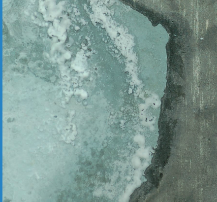
Impact of battery acid on bare steel.
